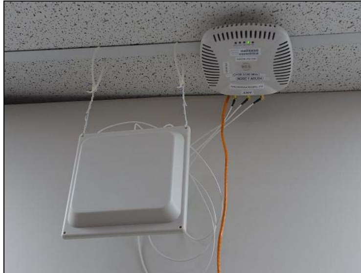
Figure 1 – Setup of Wi-Fi access point 1 (5180 MHz) near the ceiling
